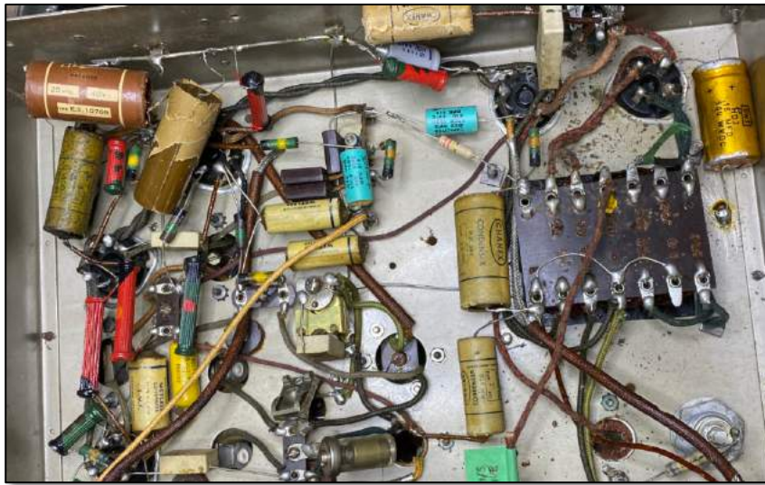
Above: An old 5 valve Scharnberg Strauss chassis undergoing re-capping, and some re-wiring.
